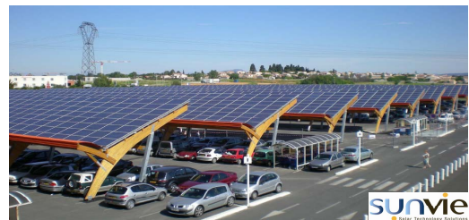
Figure 1. Car parking sheds with photovoltaic power plant.
